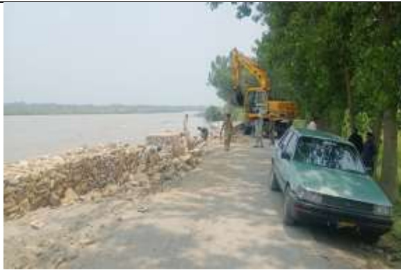
Construction Activities without PPEs and Safety measures at Package 12 (Mamu Khatki)
