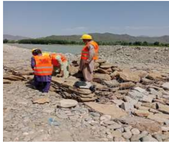
Status of PPEs Compliance at site
