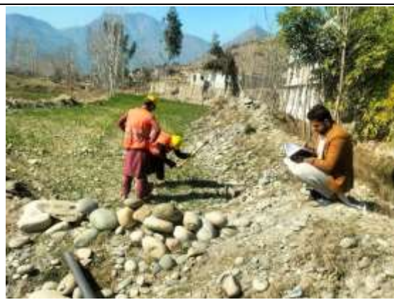
Status of PPEs Compliance at site
