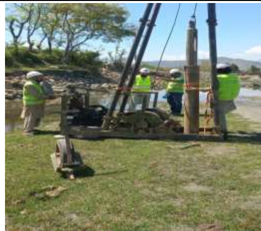
Status of PPEs Compliance at site
